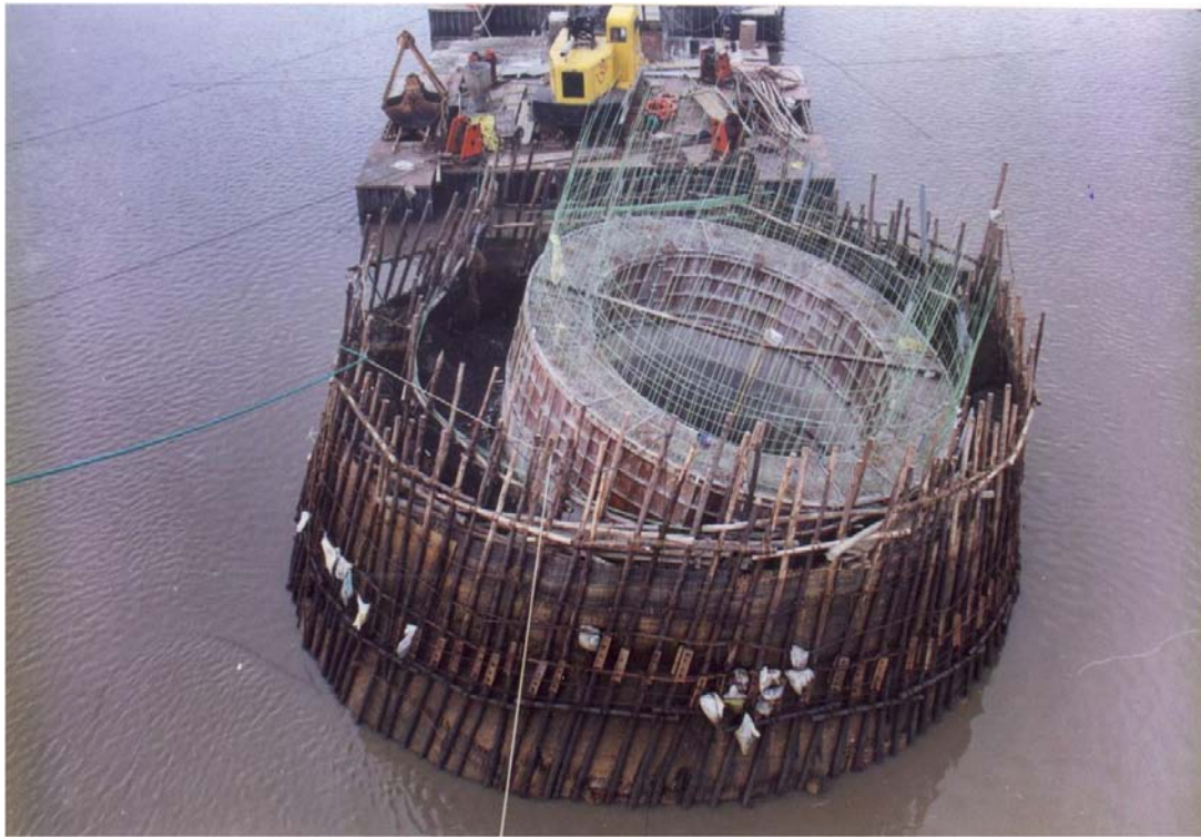
Fig 17.8 Tilted well of pier no 6 of Dharamtar Bridge
